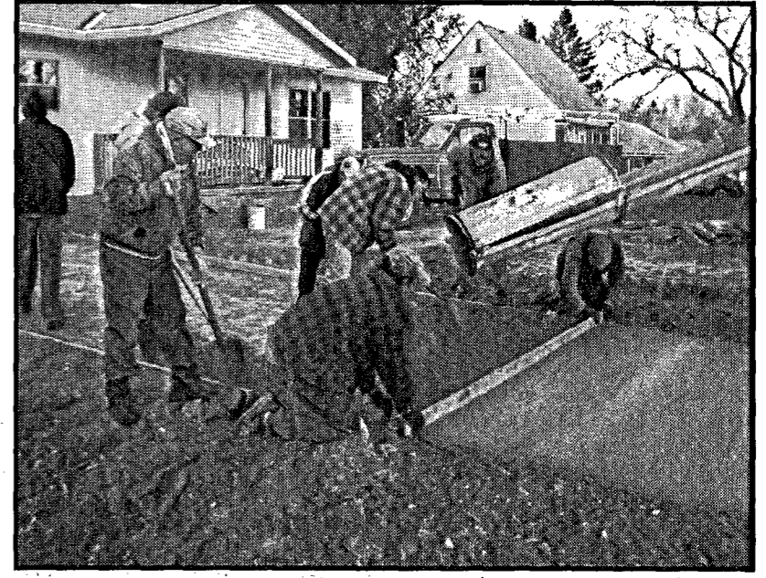
Volunteers help pour the concrete for the current Habitat for Humanity home being built in Wayne.
